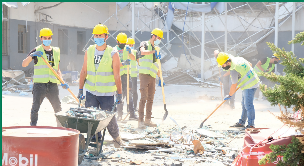
Lebanon. ILO's Employment Intensive Infrastructure Programme (EIIP) creates 200 decent jobs for Lebanese nationals and Syrian refugees, 15 per cent of whom are women, to help restore livelihoods and support the clear-up operation in Beirut. ILO Photo.
